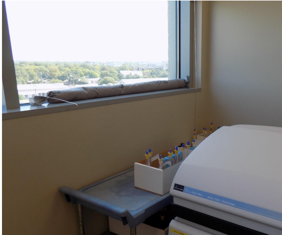
Makeshift Approaches for Protecting $250,00 Equipment from Incoming Rainwater
