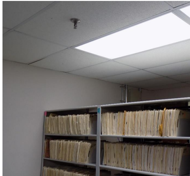
Adoption Paper Files Sit Unprotected Under Water Sprinklers
